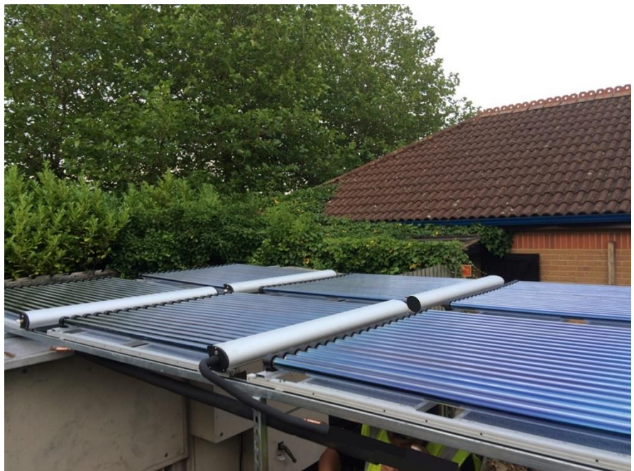
Picture 1: A Solar installation at Cummins Peterborough (Source: SCE image library)
